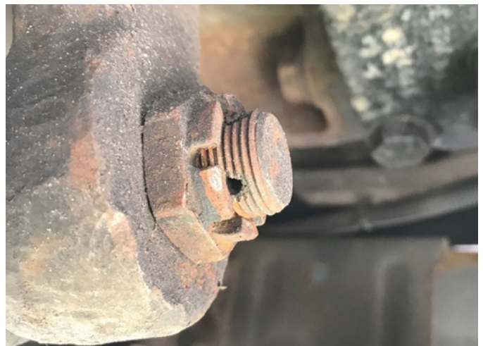
Fig 6: Missing split pin
